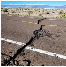
Roadway severed from NJ earthquake
